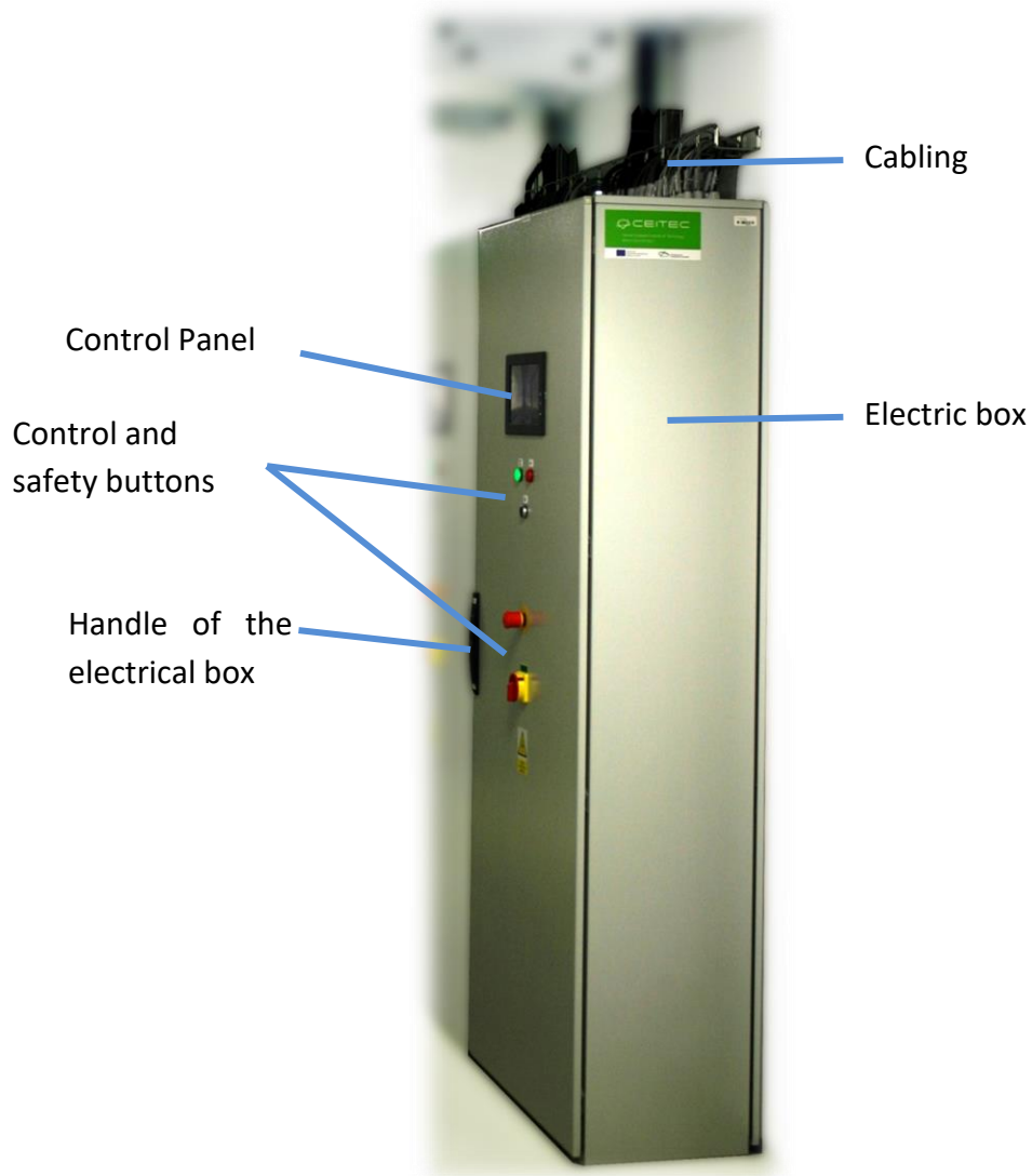
Pict. 1 Control and electrical box
